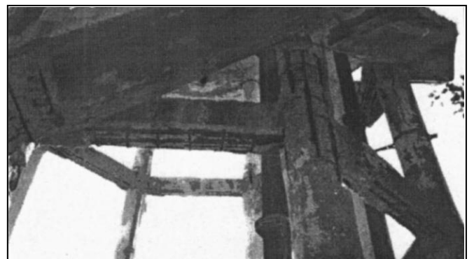
Fig. 6. Corrosion in reinforcement and spalling of concrete in bracings in water tank.
