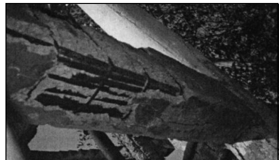
Fig. 9. Close-up of spalling of concrete in the bracing of one water tank
