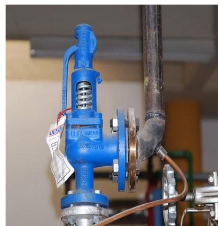
Figure 2 Boiler Safety Valve
