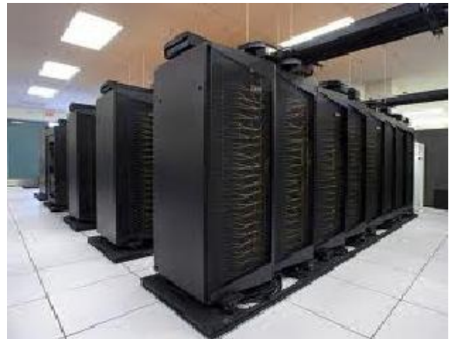
Fig. 2. Cloud Data Center
