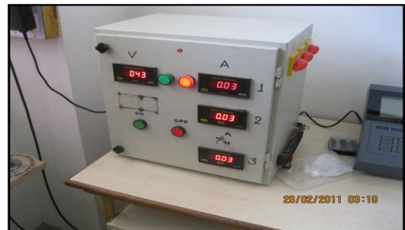
Fig-4 Photograph Of Rectifier
