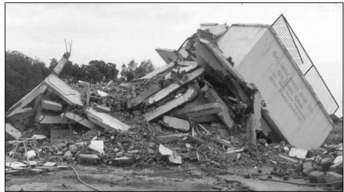
Fig. 3. Collapsed slender and weak framed stagings of water tanks in Manfera village.
