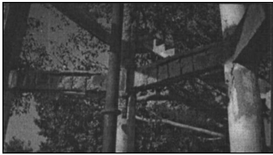
Fig. 10. Spalling of concrete and reduction of reinforcement cross section in bracing, column, and staircase of one water tank
